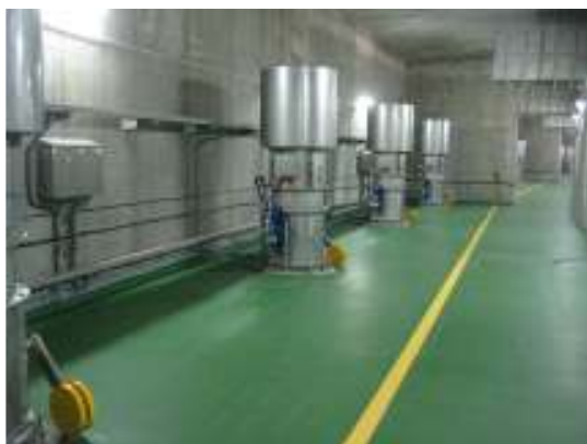
3) Inside the turbine hall – showing the Wells turbines*
